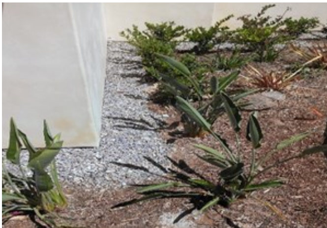
Mulch is pulled back at least 12 inches away from the structure.
